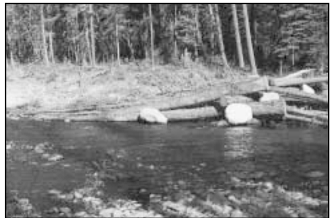
Figure 1. Debris groin at the West Kettle River, ballasted to hold ramp-logs against the channel bed.
