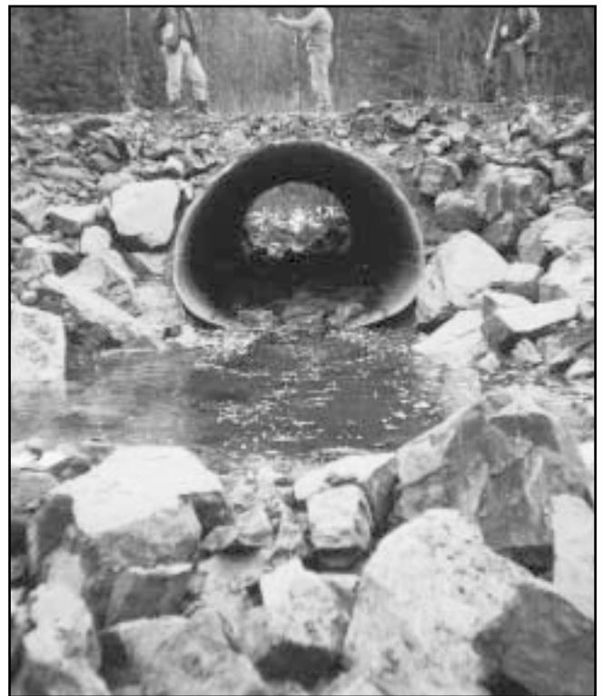
Figure 3. Before and after pictures of a culvert crossing on the a tributary to the Cottonwood River, near Quesnel B.C., for which a weir was constructed to backflood the culverts to provide fish passage.
