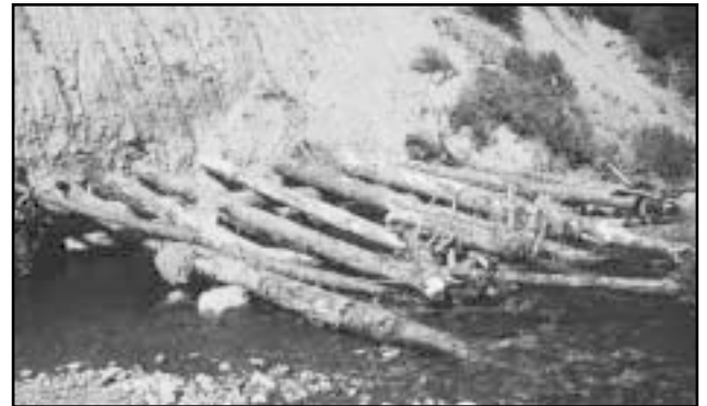
Figure 6. Debris groin located at a large steep eroding bank. Rootwads are used to gain elevation for the wide ramp of logs constructed at Narrowlake Creek.
